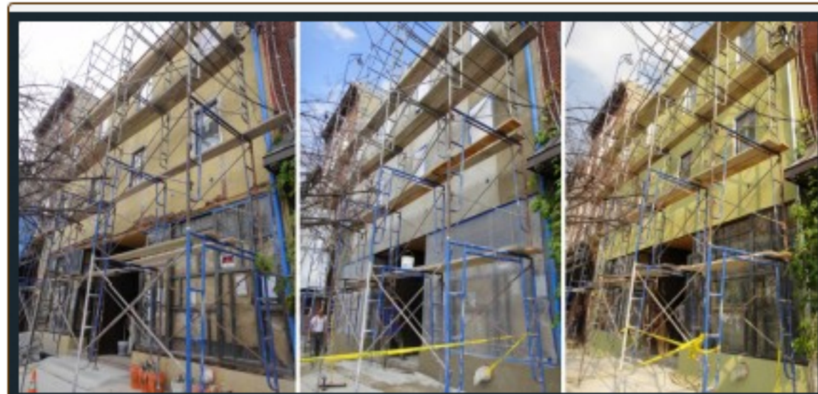
Before, during and after photos of the front of the Girard Avenue LEED-certified building of Yikes Inc.
